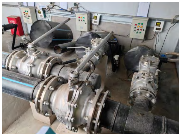
渗滤液抽取泵
